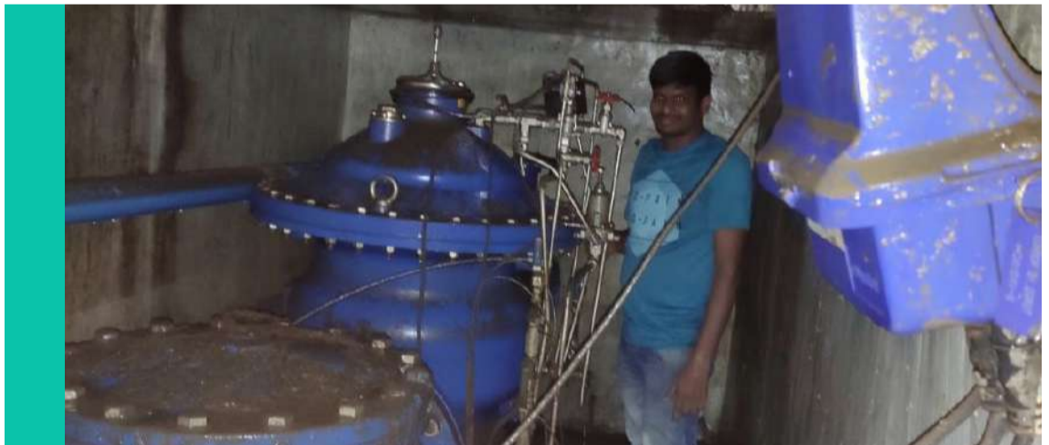
The ConDor and DOROT S300 24"/600mm valve, after the chamber had been drained.
